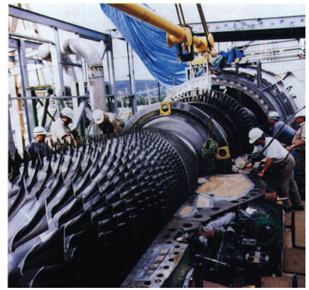
An industrial gas turbine during a major inspection event, including scheduled maintenance of servo valves
